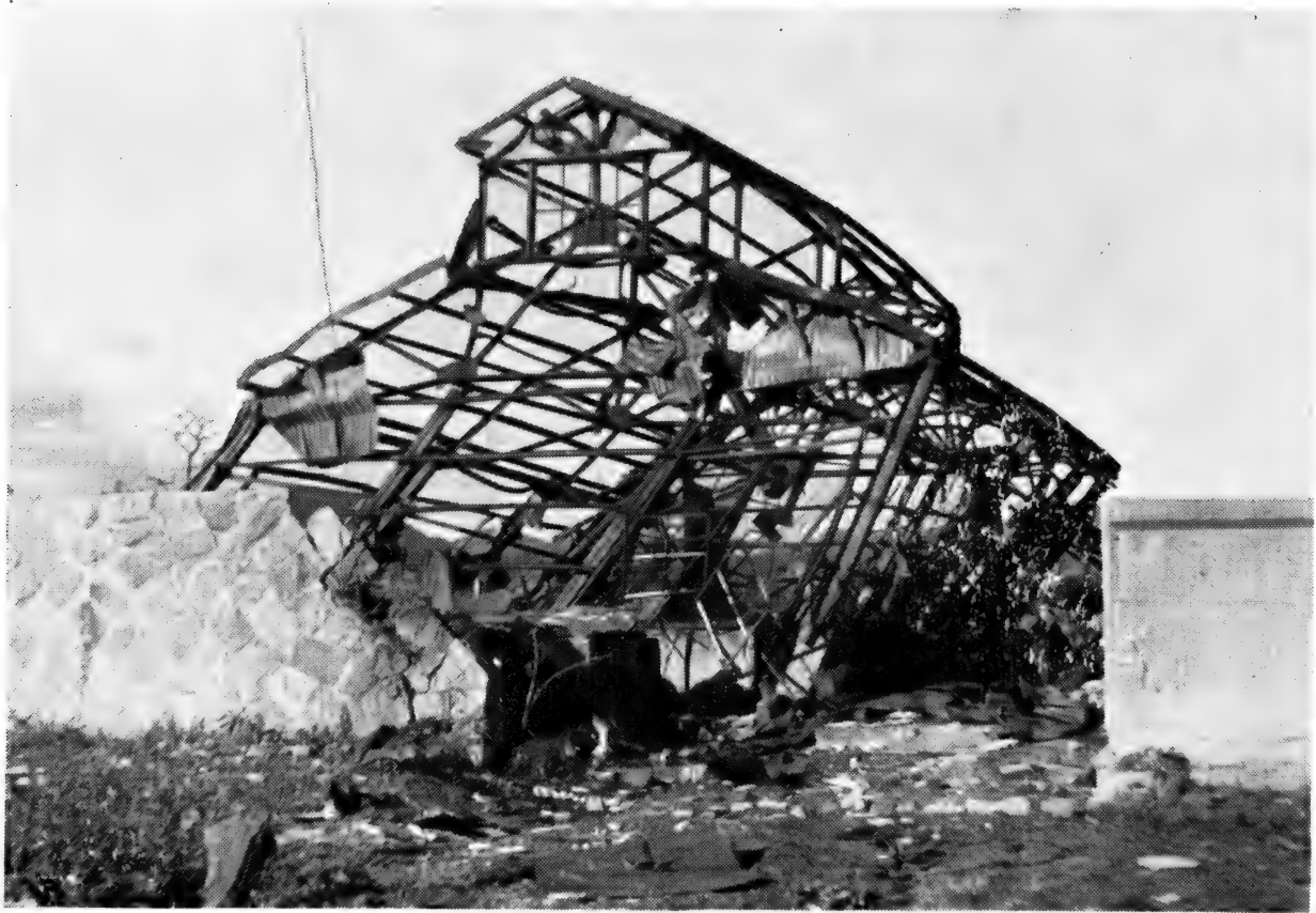
Photo No. 11. HIROSHIMA. Small steel framed shed \frac{1}{4} mile from the centre of damage, showing the distortion of the entire framework, with the building leaning away from the explosion. See paragraphs 22 and 32.
